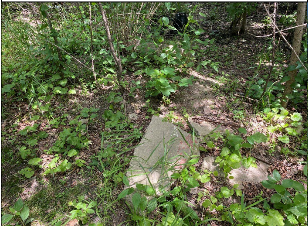
17. Partially buried concrete debris.
