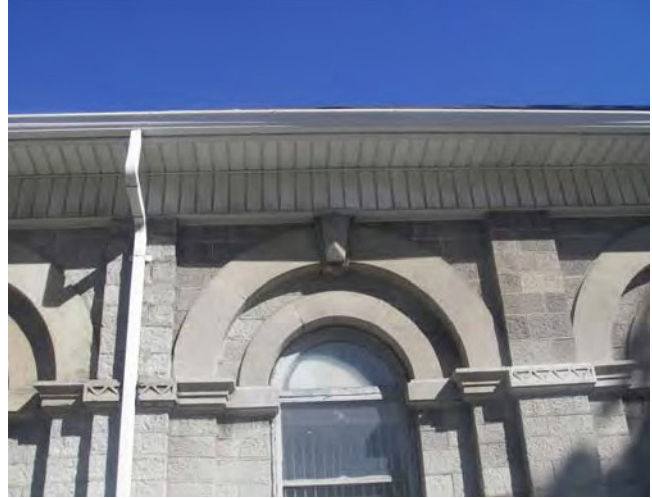
The eaves trough on the Registry Office cuts through the stone detailing of the façade. This damage is both regrettable and irreversible.
